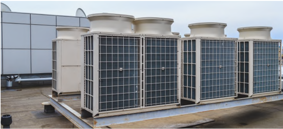
Variable Refrigerant Flow Heat Pumps
