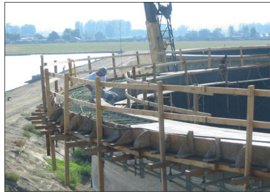
Wastewater Treatment Facility, Port of Sunnyside
