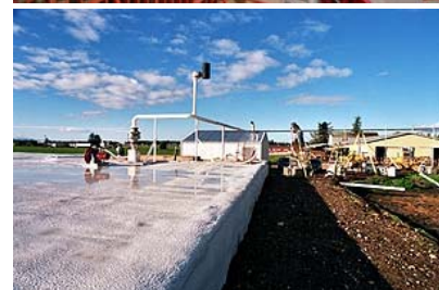
Anaerobic Digester – Vander Haak Dairy Lynden, Washington
